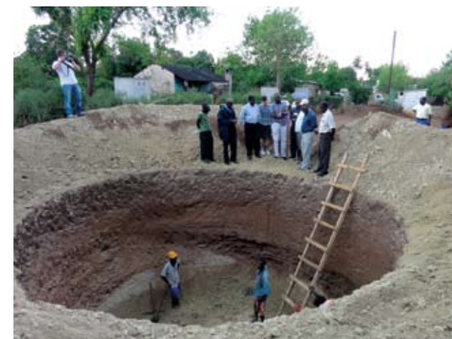
Biogas latrine construction as part of the work initiated by the Devolution Trust Fund in Libuyu, Livingstone, Zambia, November 2011.
